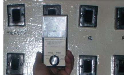
Fig. 3 Magnetometer near electrical switchboards in the office of a railway station; B = 17 mGs
